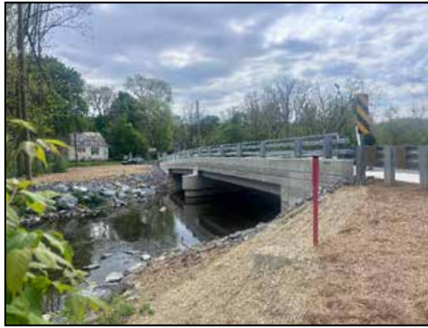
Executive Tara Zrinski. "Reopening the Meadows Road Bridge improves travel throughout Lower Saucon Township while demonstrating Northampton County's continued commitment to investing in critical infrastructure." The approximately $3.1 million bridge replacement project was funded through a reimbursement agreement with PennDOT, which covered 80 percent of the total project cost, with Northampton County funding the remaining 20 percent.
